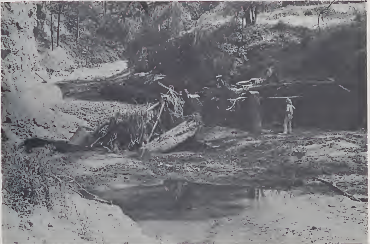
Fig. 6—Wood and concrete drop structure across Eaglehawk Creek outflanked by bank erosion. Looking upstream.
